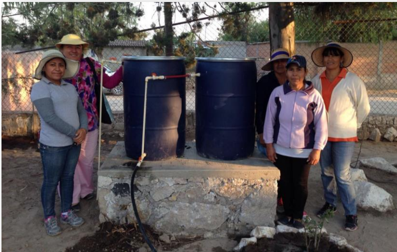
Biochar treatment system at the elementary school in Vergel de Guadalupe
