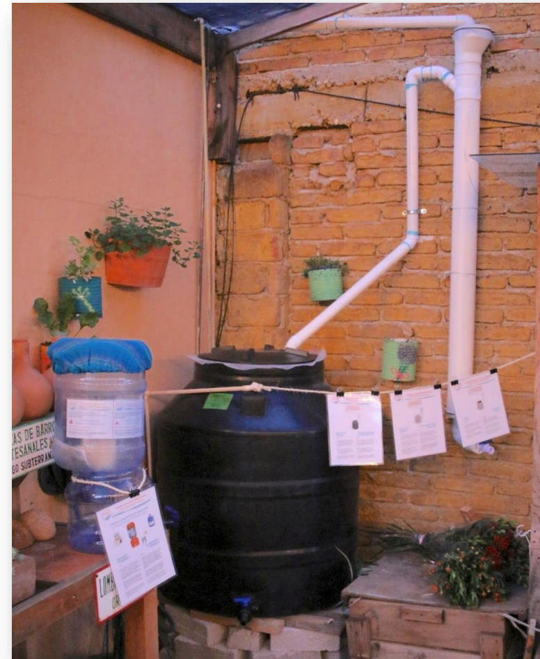
Urban Rainwater Harvesting System with Ceramic Water Filter at Vía Orgánica
